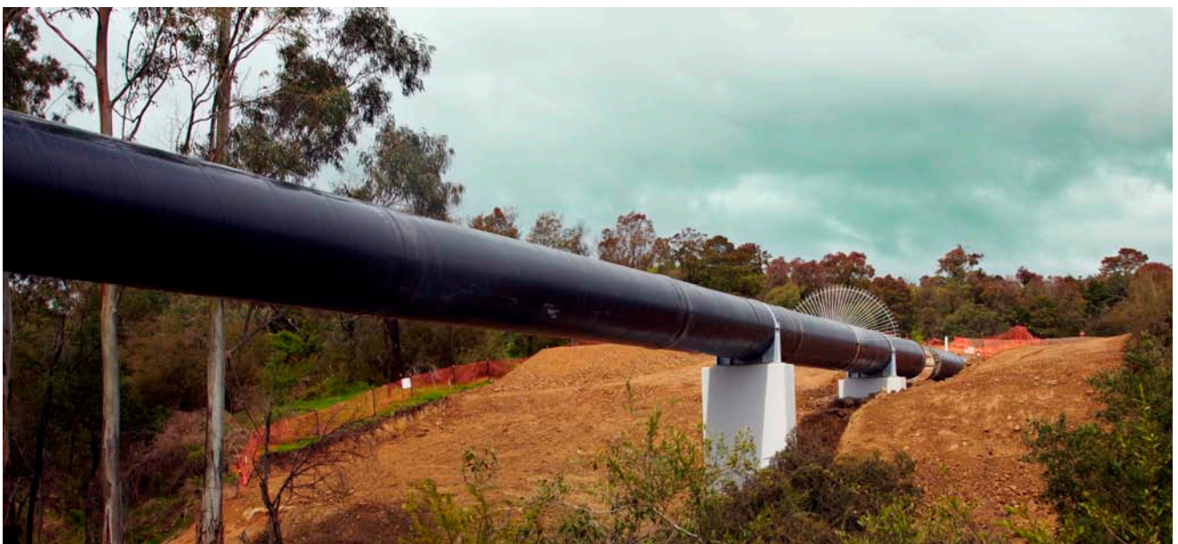
Sugarloaf Pipeline pipe bridge over the Yea River (Photo: courtesy Sugarloaf Pipeline Alliance/The Heaven Group)
