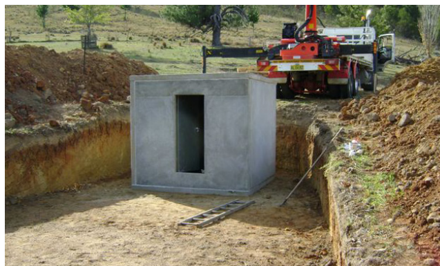
Concrete fire bunker being prepared for burial (Photo courtesy of Aussie Precast)
