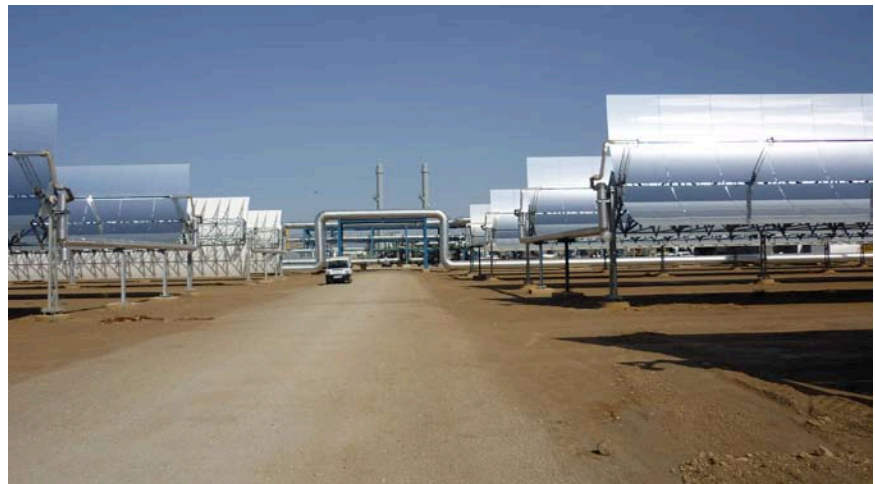
The Andasol plant is Spain's first commercial solar thermal plant with molten salt storage. The storage capacity allows it to supply power for 7.5 hours after sunset. (Photo: courtesy of Beyond Zero Emissions)
